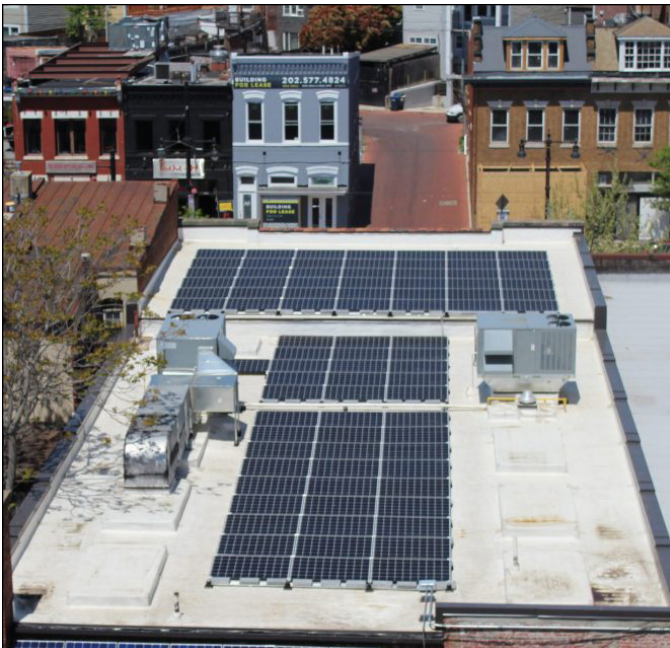
Solar panels installed on flat roofs of commercial buildings can be concealed behind parapets and remain out of view from the public right of way. Image from Ipsun Solar.
