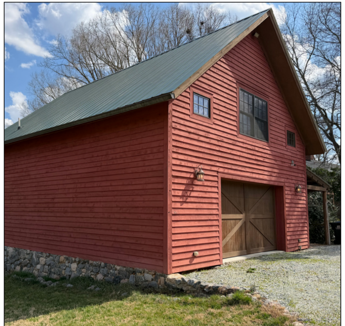
Construction of a compatible modern garage at the Thompson House near Wake Forest was a major work approved by the WCHPC. Photograph by Capital Area Preservation, Inc.
