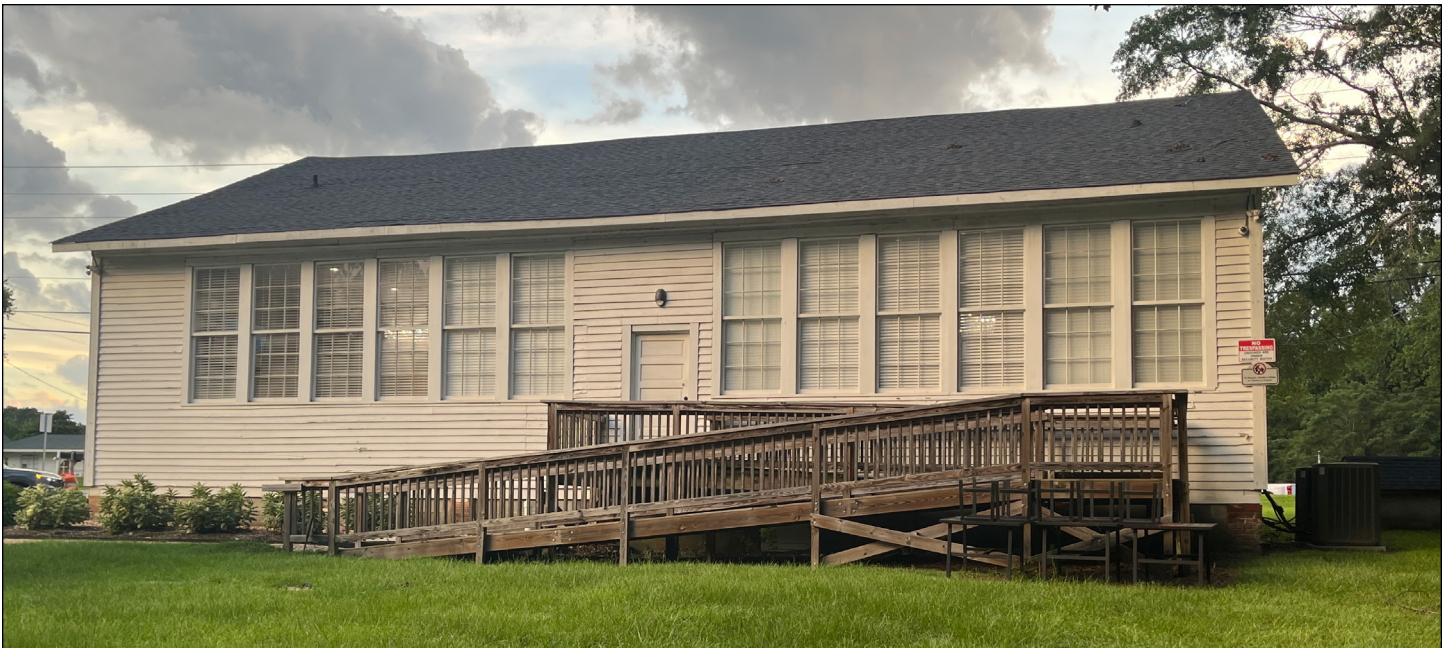
An accessibility ramp provides entry at the rear of the Panther Branch Rosenwald School, away from the primary facade. Photograph by Loggia Preservation, 2025.
