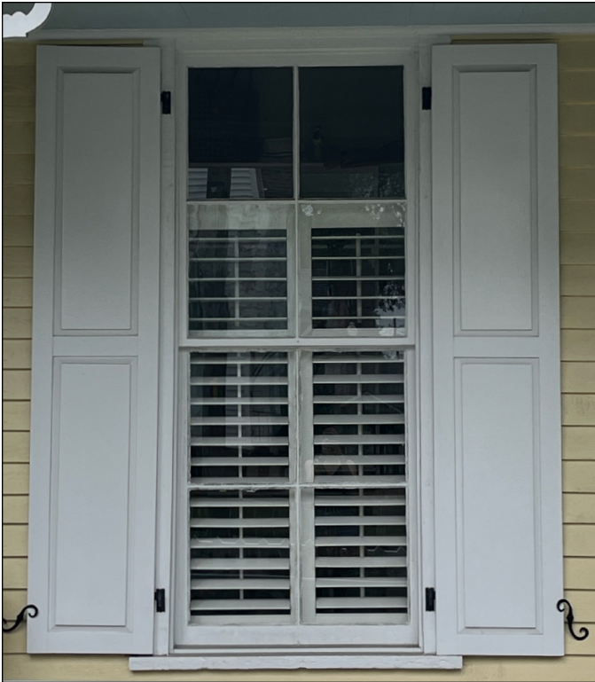
Replacement shutters at the Harward House in Apex are designed to appear operable. Photograph by Loggia Preservation, 2025.
