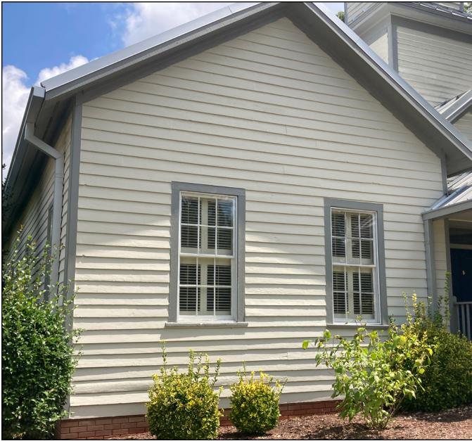
Corner boards and window trim frame exterior wall openings and define the edges of the wood siding. Photograph by Loggia Preservation, 2025.
