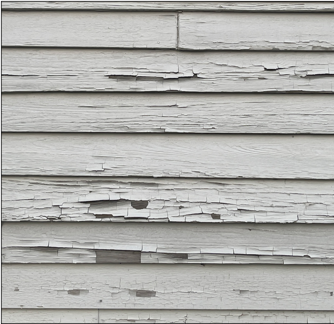
A cyclical maintenance schedule can help prevent excessive deterioration. When work is required, the repair of deteriorated wood must be prioritized over full replacement. Photograph by Loggia Preservation, 2025.
