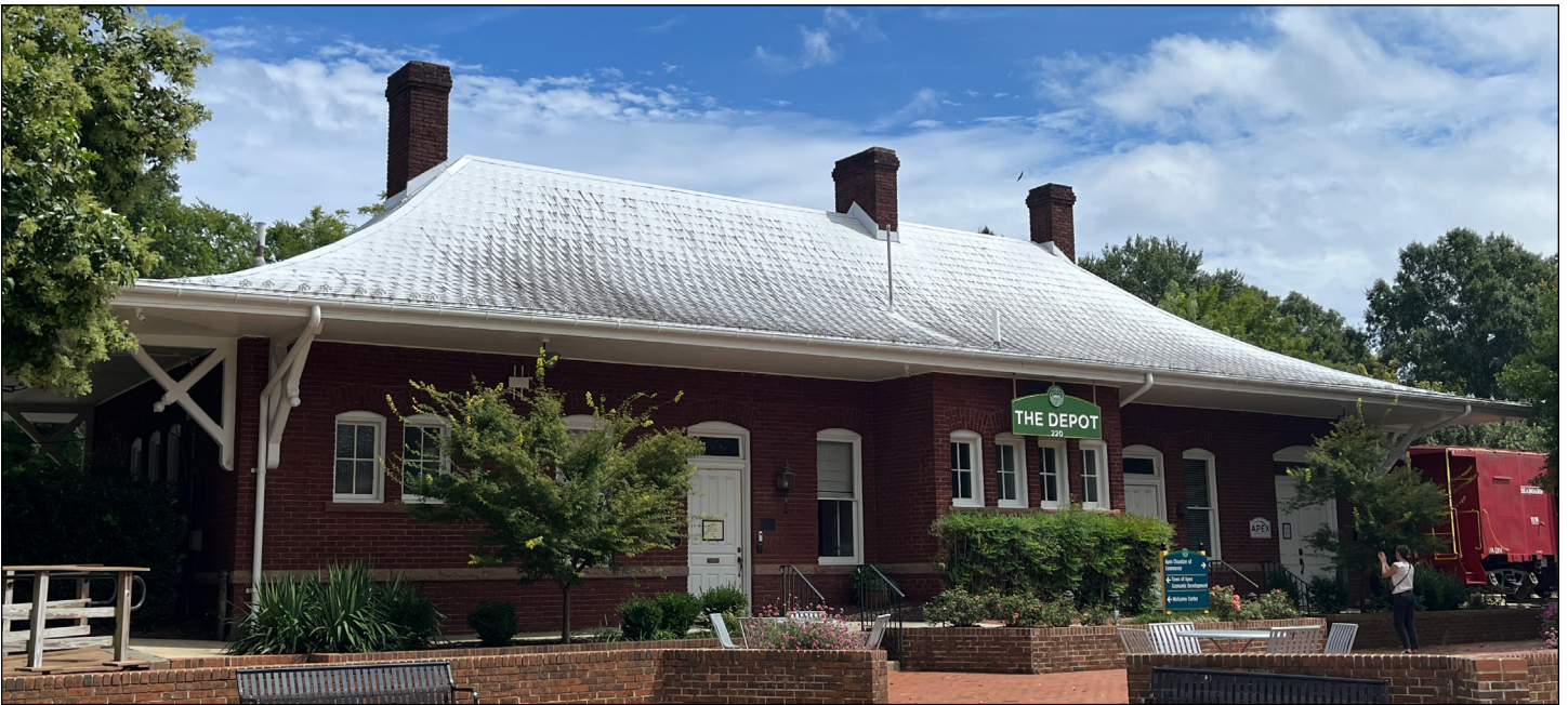
The Apex Union Depot features a distinctive bell-cast hipped roof clad in individually pressed metal shingles. Photograph by Loggia Preservation, 2025.
