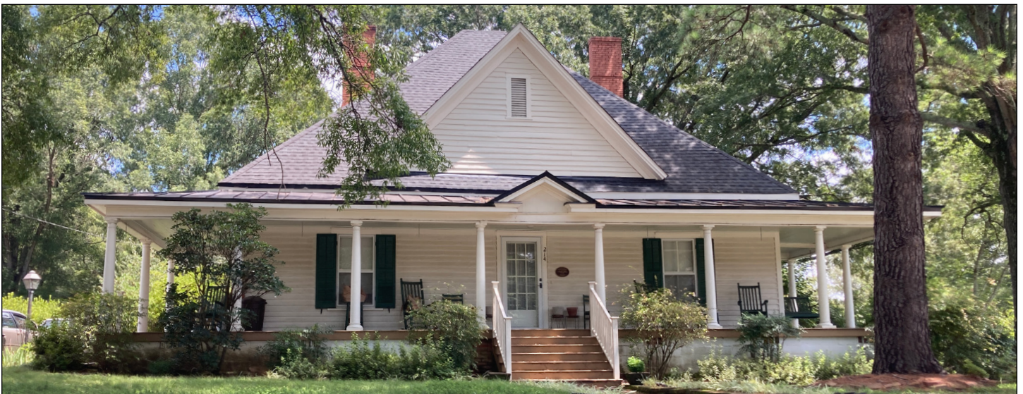
Resilient design features like the deep wraparound porch, tall roof, and elevated foundation of the Reverend Robert E. Atkins House in Morrisville illustrate historic methods for mitigating heat and weather. Photograph by Loggia Preservation, 2025.
