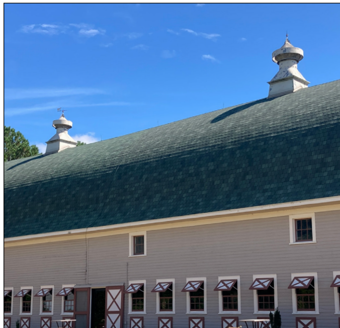
The metal cupola vents on top of the Wakefield Barn, near Wake Forest, reflect historic agricultural ventilation design. Photograph by Loggia Preservation, 2025.
