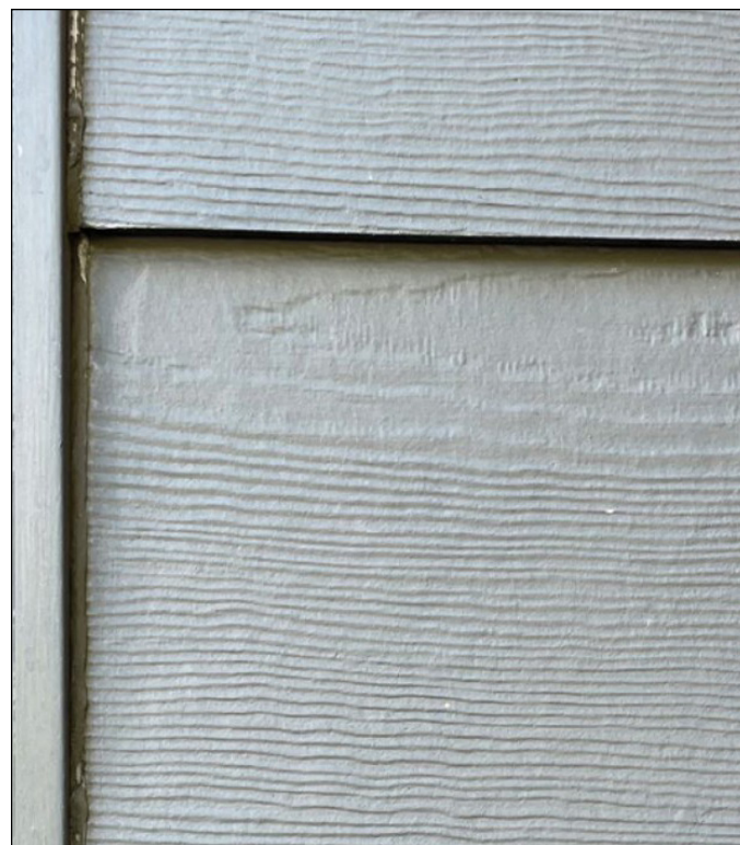
One pitfall of alternative siding material, shown here, is the surface texture. Historic wood siding has a smooth texture and does not show graining. Photograph by John Sandor in Preservation Brief 16.
