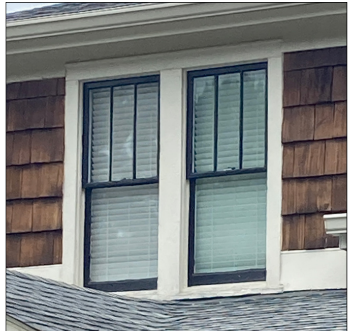
The 3-over-1 wood windows at the Craftsman-style JF and Mary Lelia Keith House in Knightdale contribute to the historic rhythm and proportion of the facade. Photograph by Loggia Preservation, 2025.
