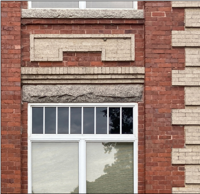
Contrasting blonde and red brick with stone lintels and sills at the Wakelon School in Zebulon constitutes a character-defining masonry feature that must be retained and preserved. Photograph by Loggia Preservation, 2025.
