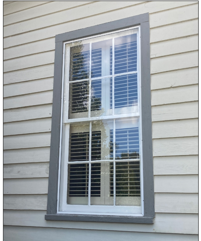
Reversible interventions, such as the storm windows shown here, can be installed without permanently altering the historic fabric. Photograph by Loggia Preservation, 2025.
