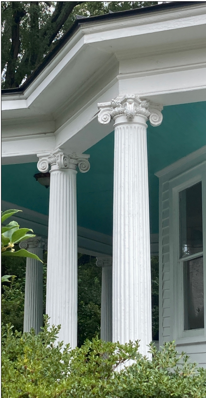
Porch detail from the Walter-Aiken House in Fuquay-Varina. Photograph by Loggia Preservation, 2025.
