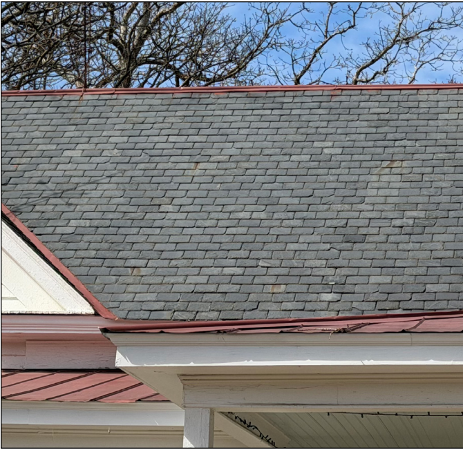
The decorative slate roof at the Wayland E. Poole House near Garner highlights the use of patterned slate as an ornamental architectural feature. Photograph by Capital Area Preservation, Inc.
