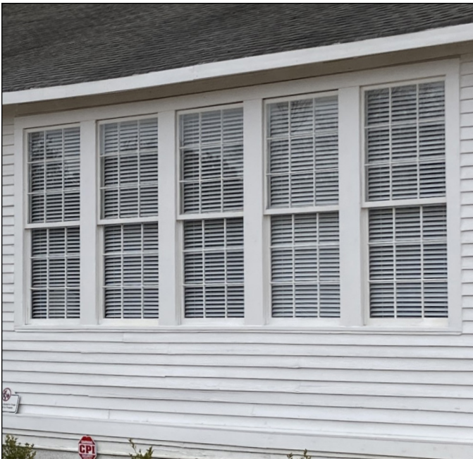
The large 9-over-9 wood windows at the Panther Branch Rosenwald School maximize natural light while defining the building's historic educational design. Photograph by Capital Area Preservation, Inc.
