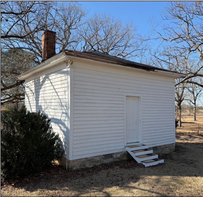
Historic preservation is not limited to grand architecture. Modest buildings, such as the office building at the Joseph Blake Farm in Shotwell, convey important history about the site. Photograph by Capital Area Preservation, Inc.
