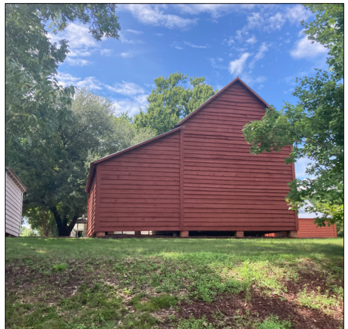
An outbuilding at the Seagroves Farm in Apex. Photograph by Loggia Preservation, 2025.
