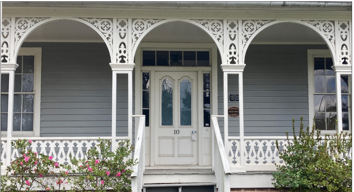
The Pugh House in Morrisville features a decorative porch balustrade, columns, and spandrels that help convey its historic character. Photograph by Loggia Preservation, 2025.
