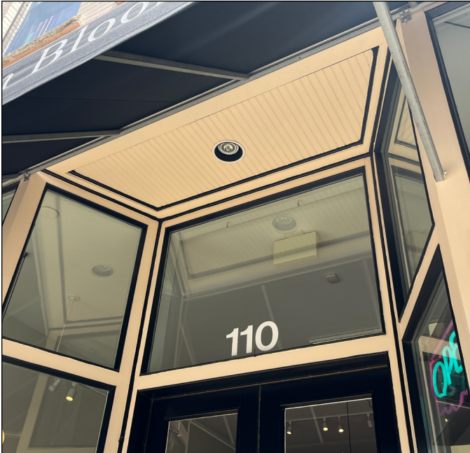
Transom windows above the storefront entrance at the Sellars Building in Apex allow abundant natural light to flood the interior. Photograph by Loggia Preservation, 2025.
