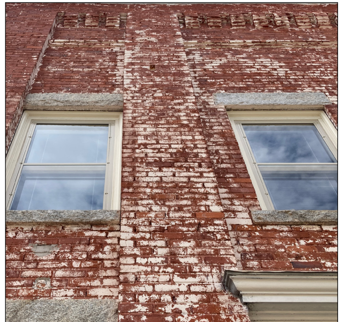
Painting previously-unpainted historic brick is not appropriate. Coatings trap moisture and accelerate spalling and mortar deterioration. Photograph by Loggia Preservation, 2025.
